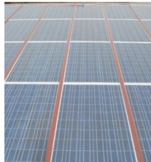
28 kWp Firenzuola (FI)
