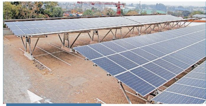
Bidco oil refineries Kenya- 1500 KWP Plant
